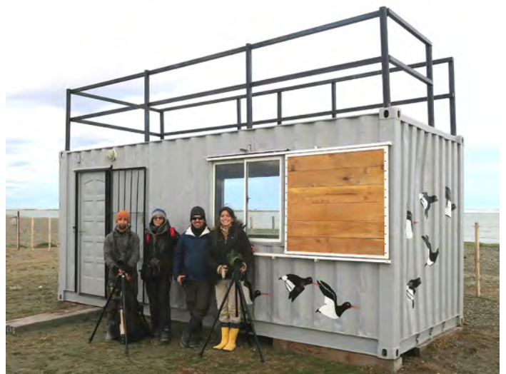
Reserve guards in front of the new ranger station and bird observation platform made from a shipping container at the Rio Gallegos Provincial Reserve. Photo: Scott Hecker
